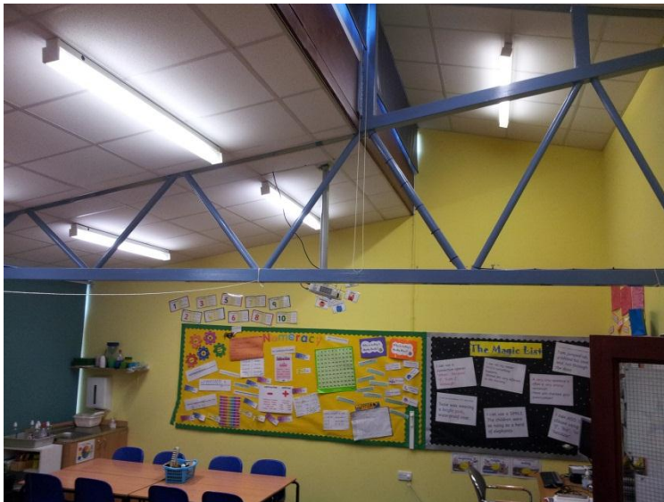
T8 switch-start batten-fittings (5ft using approx. 70Watts)
