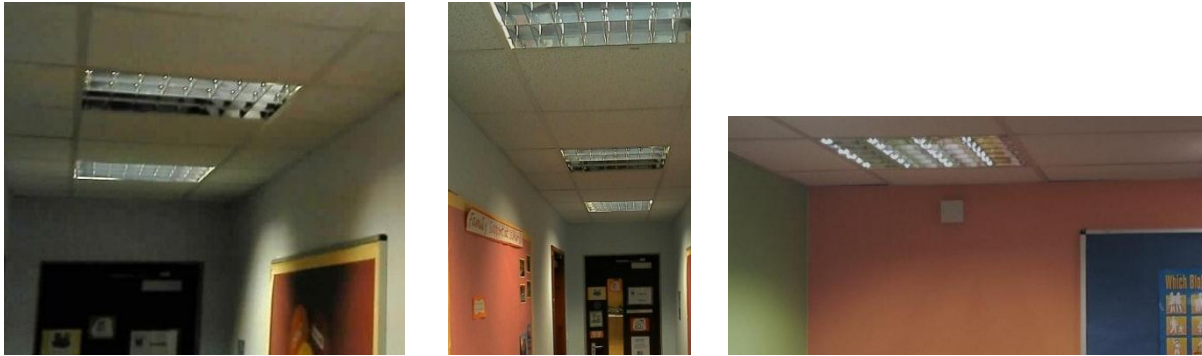
'Cat2' modular lighting showing 'cave' effect (each lighting using approx. 90 Watts)
